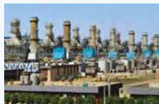
Suleymaniyah Combined Cycle Power Plant - Iraq
