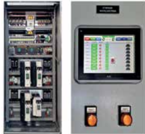
Automatic Control System
