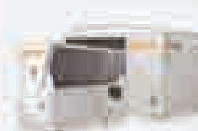
▶ Air Handling Units
